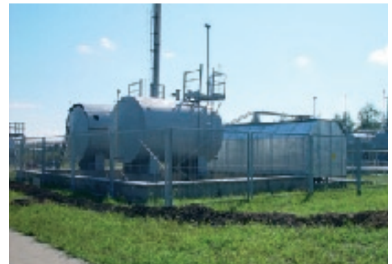
| photo 16 | Compact complex gas treatment plant for small gas-condensate fields
