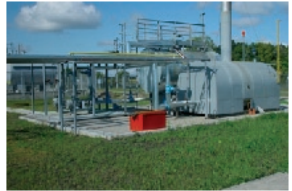
| photo 15 | Compact complex gas treatment plant for small gas-condensate fields
