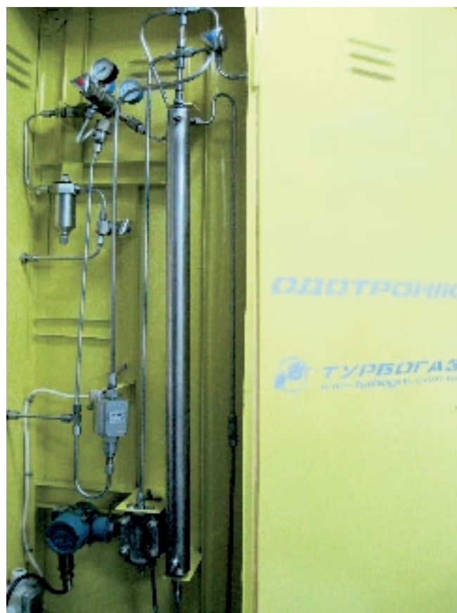
| photo 14 | Gas odorization system "ODOTRONIC"
