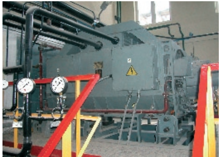
| photo 3.1 | Generator UDEU – 2500 – UHL4
